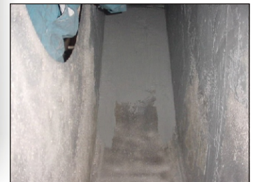
Interior was severely eroded, with many holes penetrating the walls. DurAlloy was used to rebuild all surfaces.
