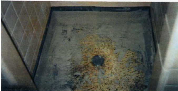
Leaking existing terrazzo shower pan. Note tape applied above the first course of tiles to neatly define the DuraQuartz repair.
