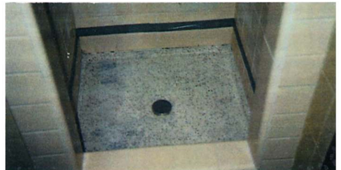
After all the surfaces to be protected are primed, the ENECRETE DuraQuartz application begins.
