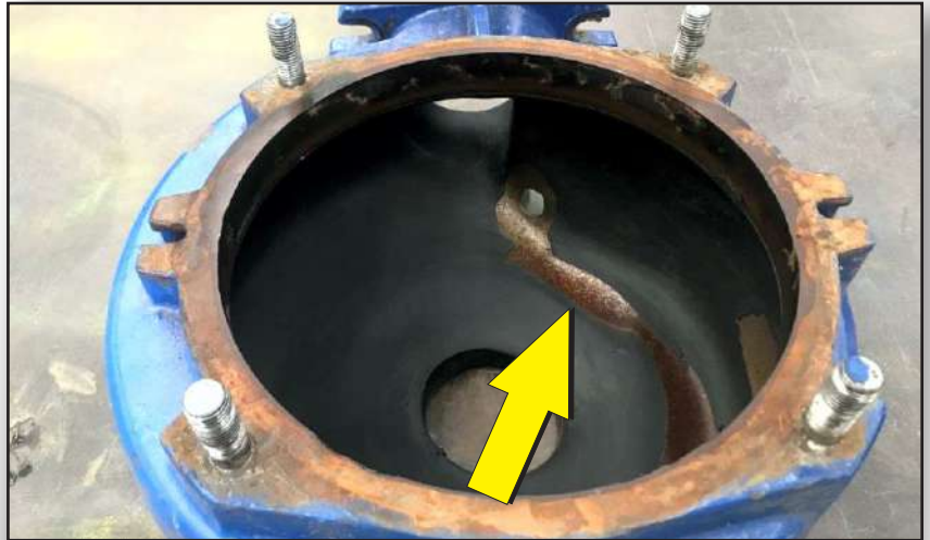
Failed rubber liner after 8 months
